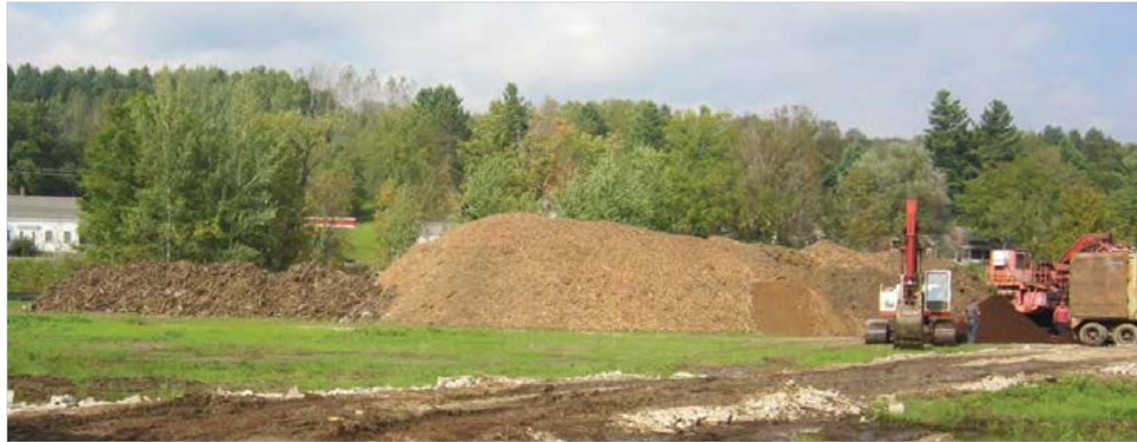
Above: Wooden remnants were fed into a huge tub grinder which reduced them to coarse mulch. The pile on the right was the building after its first pass through the grinder. On the left were the remains of the Somerset pipeline pieces that Haynes did not sell.
